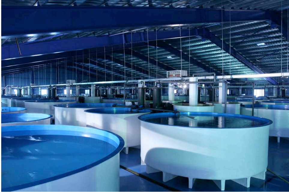
Figure 9: Cell Aquaculture Tanks, Terengganu, Malaysia (Photo courtesy of Cell Aquaculture, 2008)
