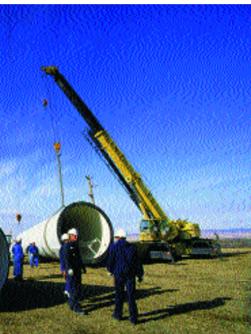
Construction of a wind turbine in Southern Alberta. (Photo: courtesy Vision Quest Windelectric Inc.)
